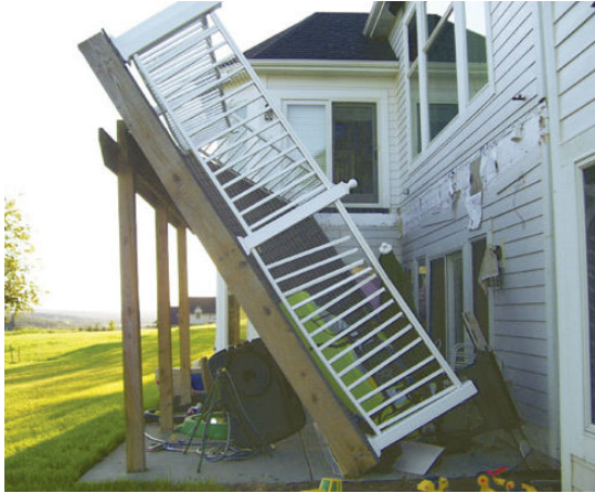
Typical deck collapse due to corroded fasteners
